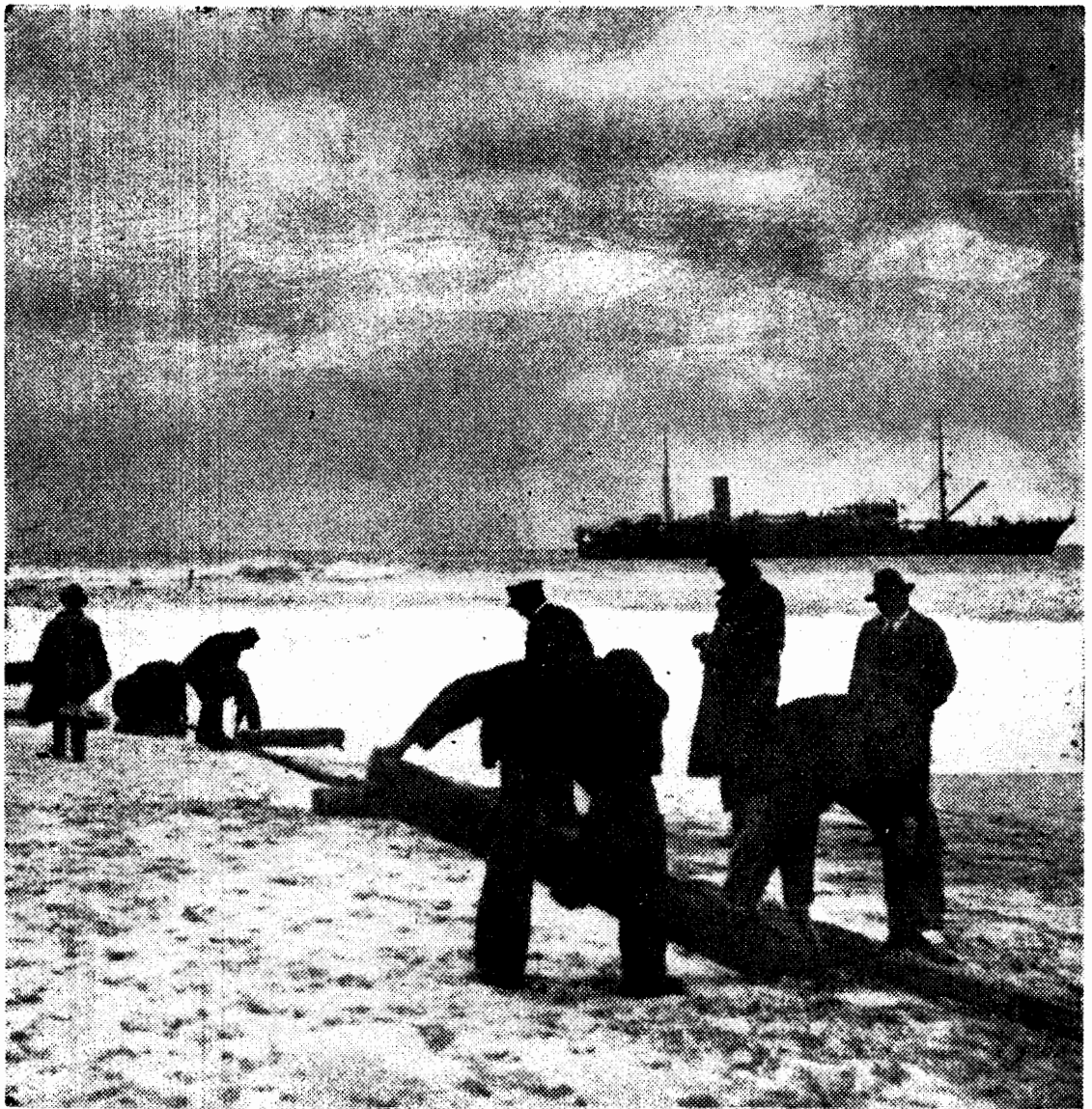
A P.M.G. team securing an underwater cable on the shore of Apollo Bay, Vic.
